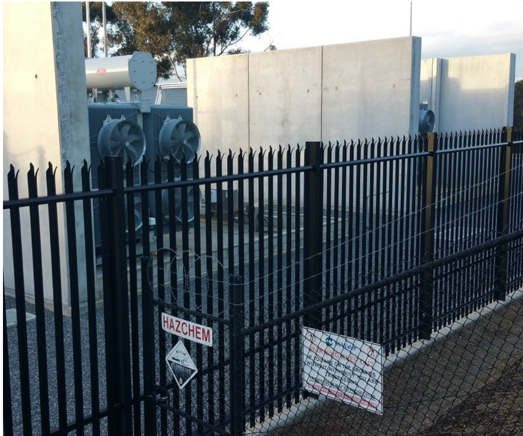
The SA Water pumping station on land stolen from Kangatilla (Park 4) opposite the Piccadilly Cinemas.
