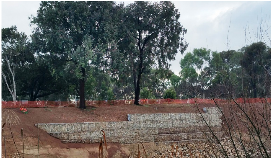
The new rock retaining walls on the cliff face, completed a little further upstream
