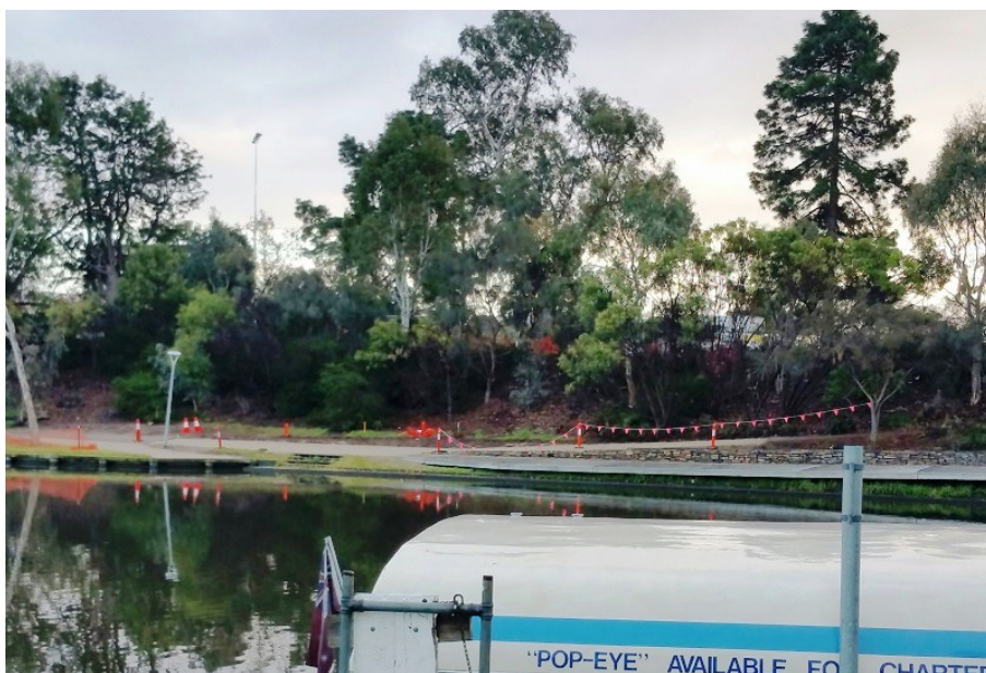
Likewise, the nearly year-long program of riverbank and footpath stabilisation works in Karrawirra (Park 12) near Angas Gardens is also nearing completion. Work has required new pilings on the
