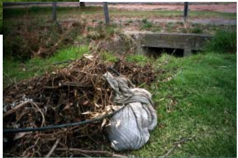
Below: Debris collected from just one small culvert.
